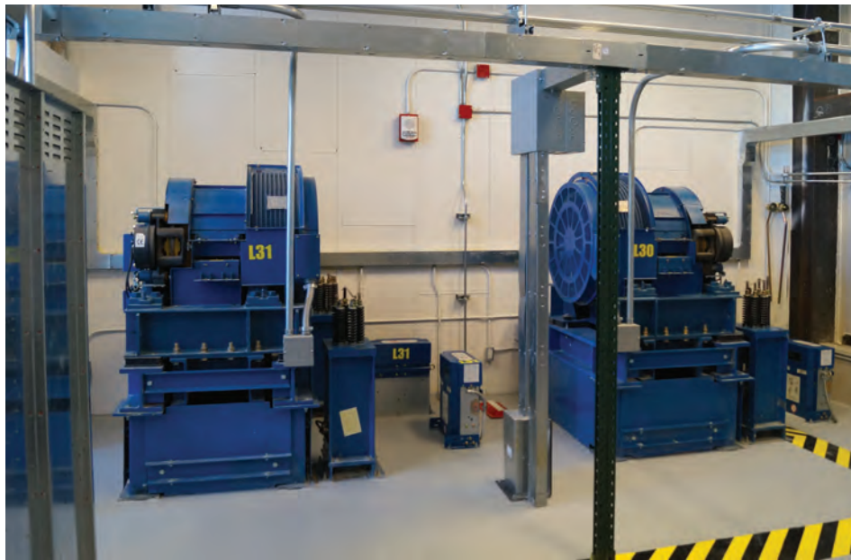
The high-rise service-elevator hoist machine, which has a capacity of 5000 lb. (2,268 kg) and a rated speed of 1000 fpm (5.08 mps).
